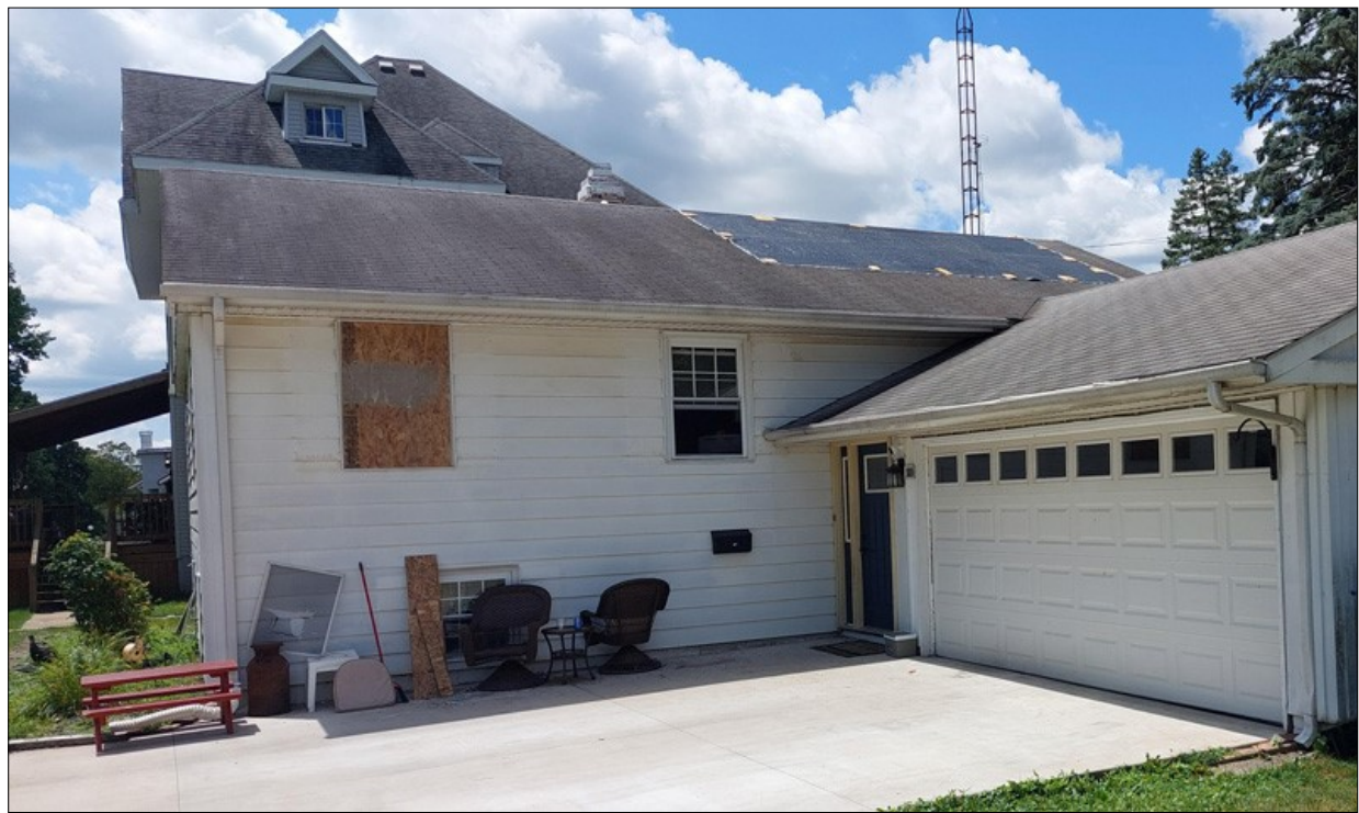
A boarded up window and tarped roof show outward signs of a house fire that caused major damage for a Hoopeston family Wednesday evening.
