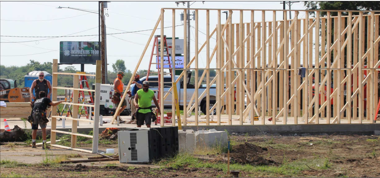
Going up Construction crews erect studs for the new Subway Tuesday morning. The restaurant will be on the southwest corner of Rtes. 1 and 9. Originally planned to be in the former First Farmers Bank building, plans changed to demolish that building and construct a new one.
