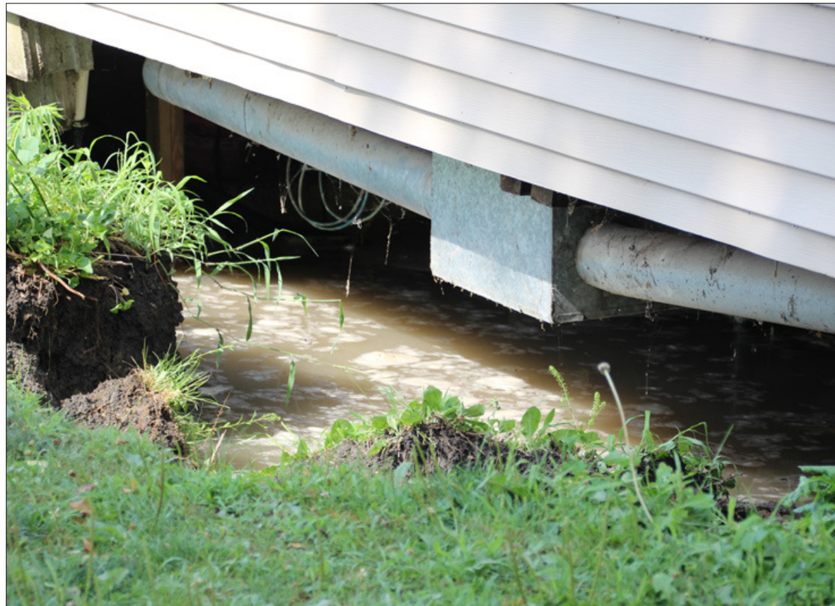
Ductwork is exposed after part of the foundation wall at 112 E. Lincoln was pushed into the basement during Sunday’s torrential rain from back-to-back severe thunderstorms.
