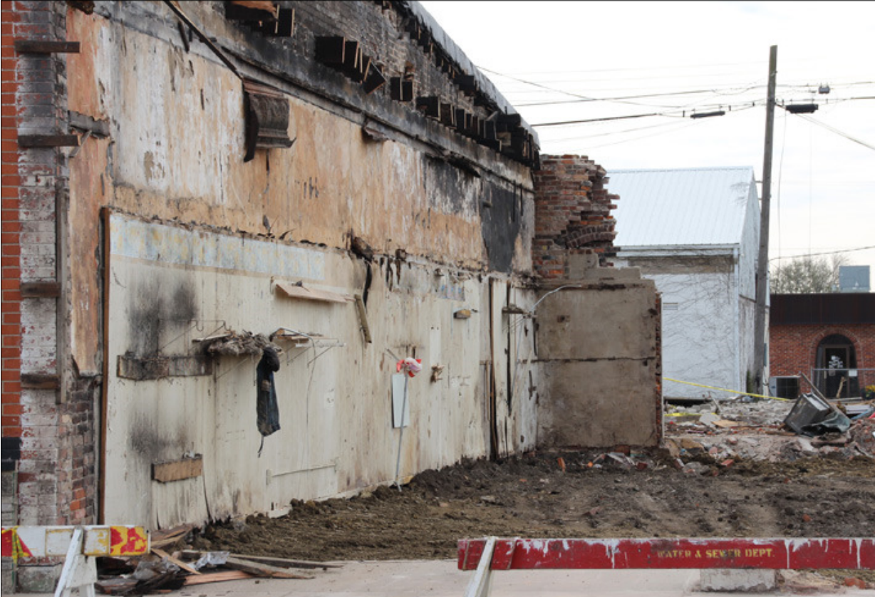
The west-facing wall of Corn Town Auctions, 109 E. Main, remains standing after 107 E. Main was torn down last week.
