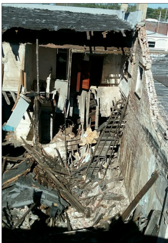
Photo contributed An aerial view shows the inside of 105 E. Main after the roof caved in on October 11.
