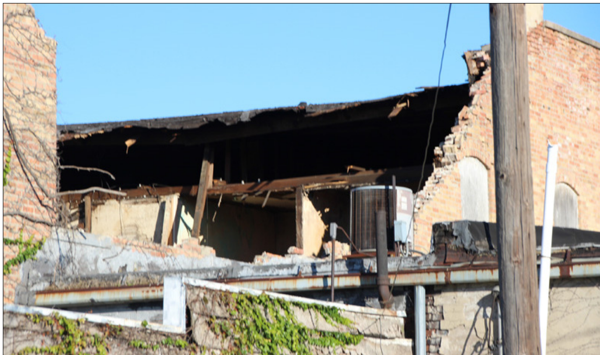
The rear view of 105 E. Main shows the exposed exterior after the roof caved in on October 11.
