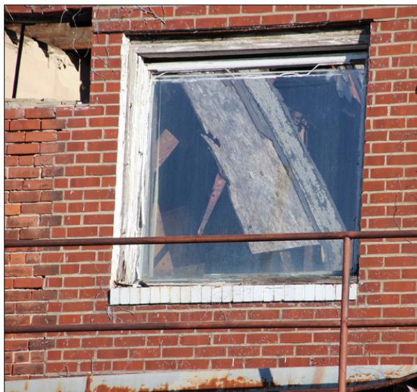
Roof debris can be seen through a rear window of the building at 105 E. Main. The roof fell through the building on October 11. The structure has been cordoned off and Main Street has been closed at the location since then.
