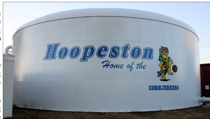
Hoopeston's ground water storage tank recently received a fresh coat of paint and the iconic Jerky. The water tower rehabilitation project is almost completed.
