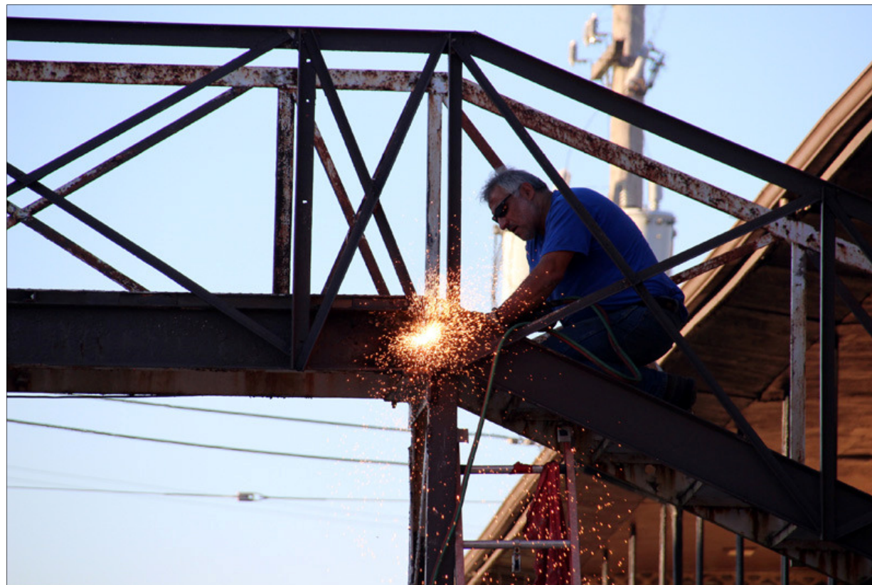
John Kincade, of Sheldon, cuts through steel to take down the catwalk between the east and west sides of the Downtown Motel Sunday evening.
