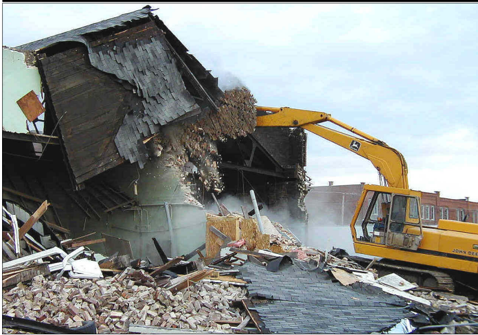
A bit of history gone Bob Voyles of Voyles Construction, Wellington, razes the former Hoopeston water building on Main Street Tuesday. The structure was built in 1897. It was severely damaged in the July 7 storm that swept through the city. City officials are planning a new building. Photo by Lourdine Florek
